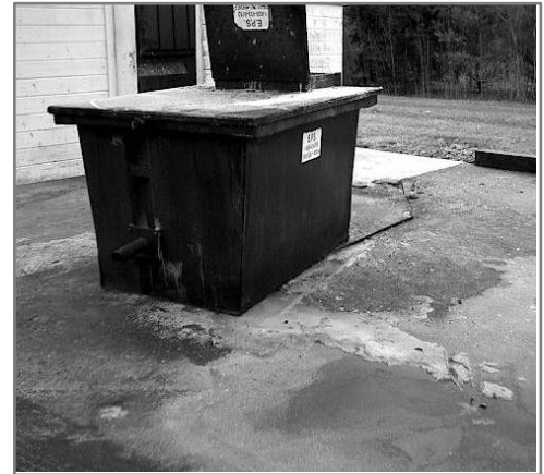
DON'T have poor grease waste management that will allow grease and other waste to accumulate on the parking lot and reach the storm drain.
