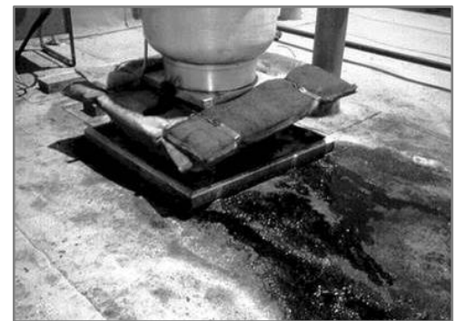
Grease from this restaurant exceeded the exhaust fan's collection capacity and eventually entered the storm water drain. DON'T let this happen at your business.
